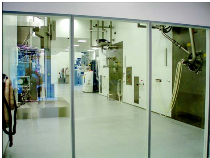
Single containment module.
